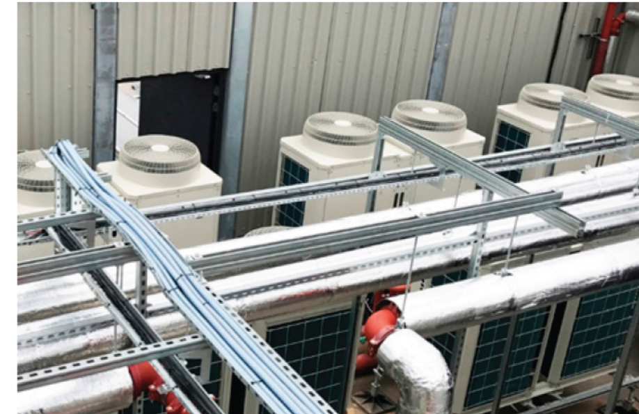
Figure A.56: Air Source Heat Pumps
