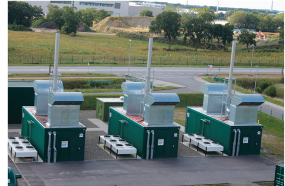
Figure A.55: CHP Generator
